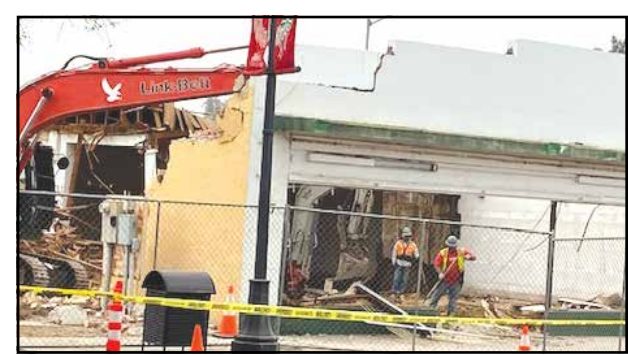
Two workers assist in demolishing the building at Highway 43 and Central Avenue which last housed the Super Discount Center, a structure with historical significance to Shafter's early days.
